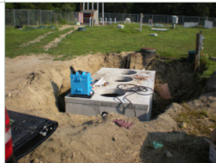
The MBR unit in this 500-gallon-per-day BioBarrier system uses micro- and ultrafiltration to process blackwater into water suitable for non-potable reuse.
