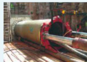
The project River Enz culvert in Pforzheim, Germany received the German Society for Trenchless Technologies Gold Award in 2011.
